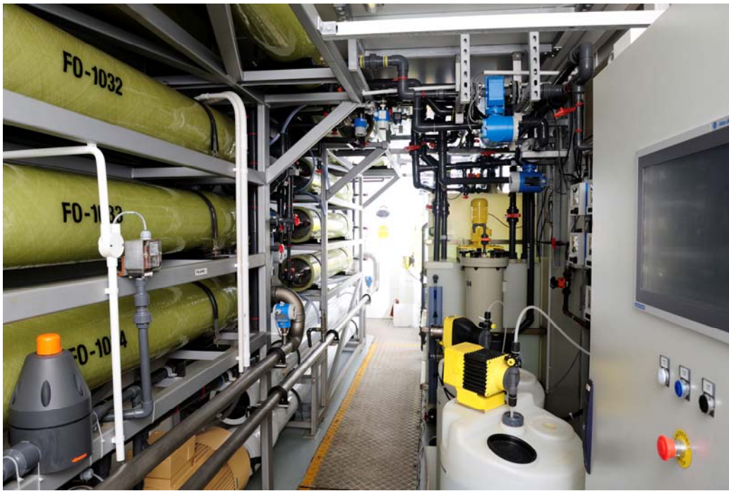
Figure 4: Inside the Process Container at Al Khaluf
