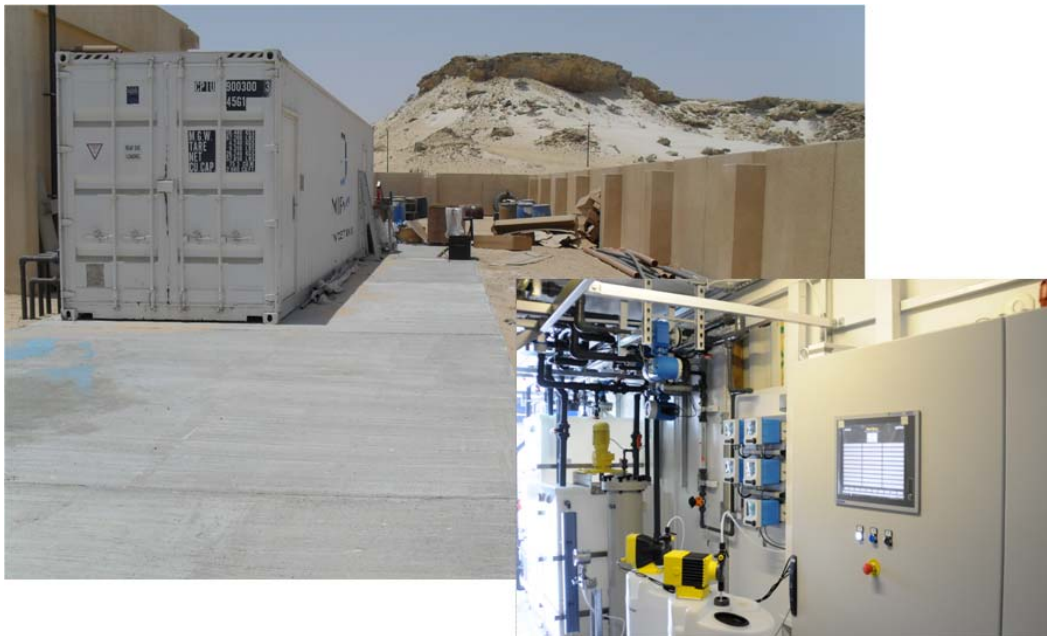
Figure 10 - The Modern Water Plant at Al Khaluf
