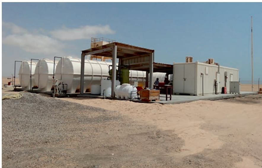
Figure 5. AI Najdah 200 m 3 /day FO Desalination Plant
