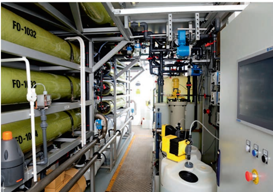
Figure 4. Inside the process container at Al Khaluf
